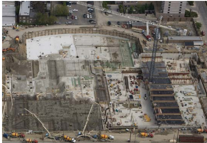
May 2007 - Four concrete pump trucks poured more than 4,000 cubic yards of concrete in less than 12 hours for the structure's hydraulic slab.
