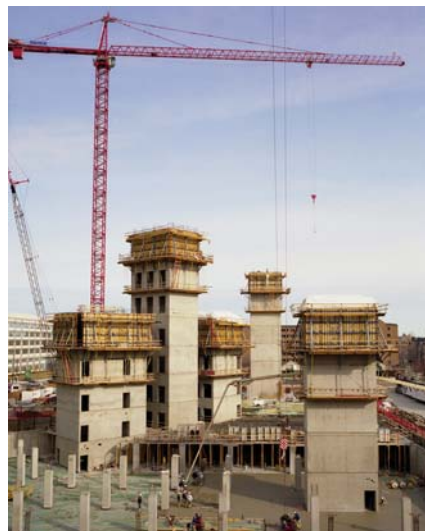
Donley's completed the concrete work for the Clinic's new Heart Center in June 2006.
